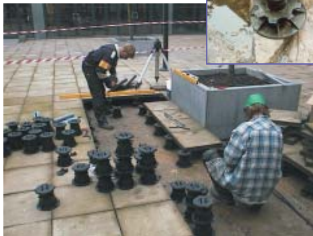
Damaged lesser quality screwjack-pedestals have all been replaced with second generation DPH5 screwjack-pedestals.
